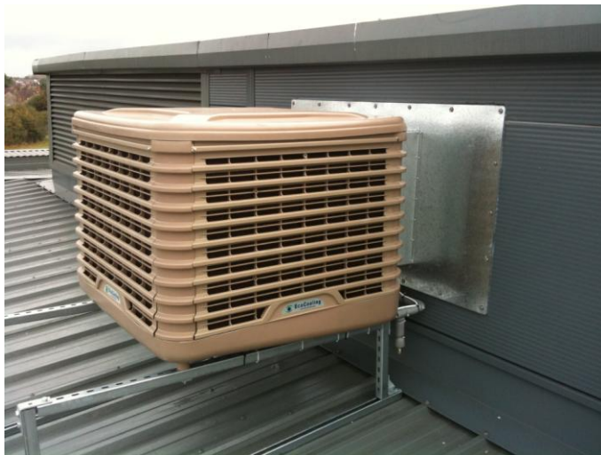
Air intake with the EcoCooling unit fitted.
